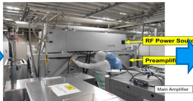
1st Amplifier installation in 2015
